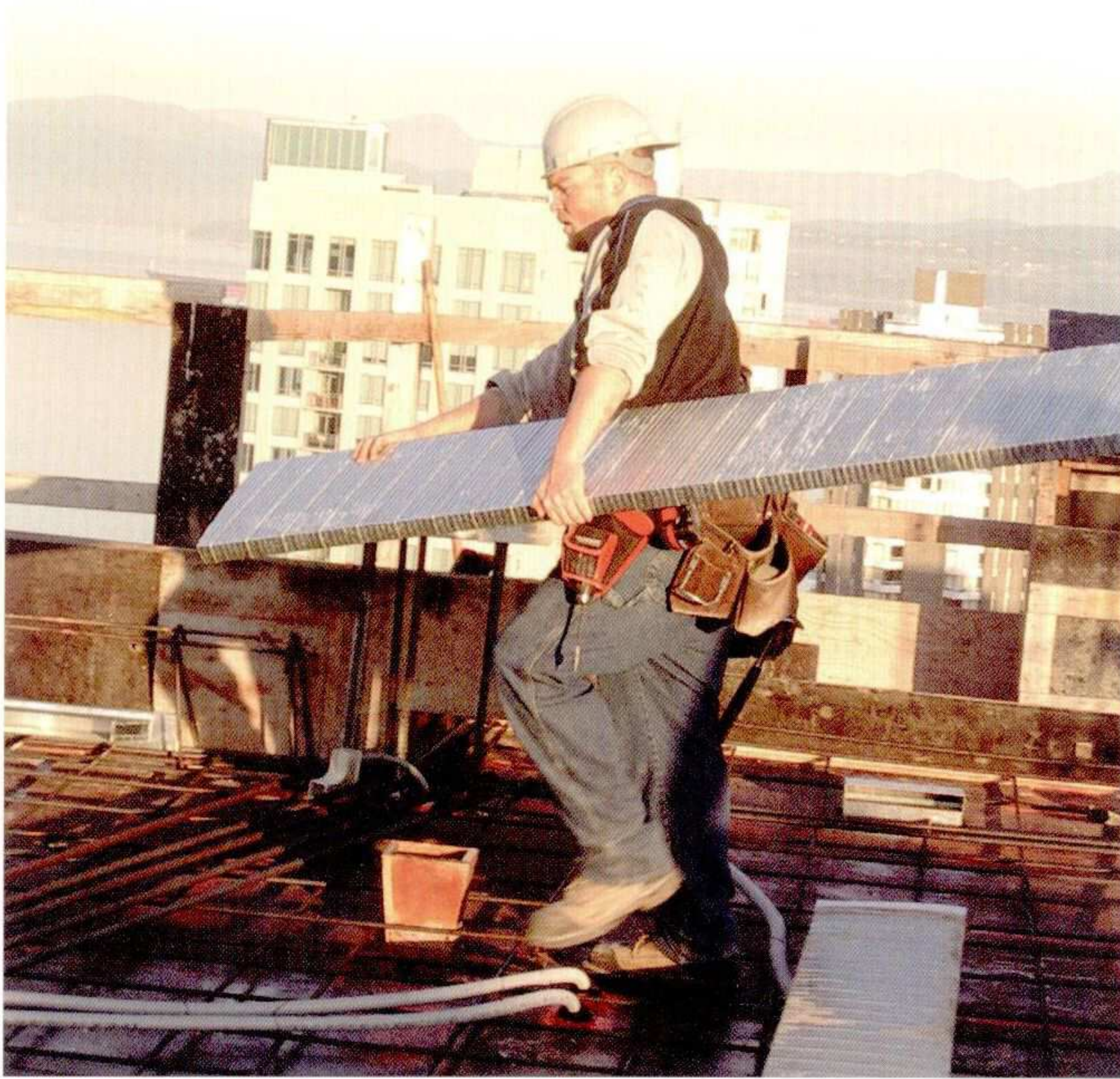
Opposite page & this page: Workers at the Pomaria site. Photos courtesy of Summit Sheet Metal.
